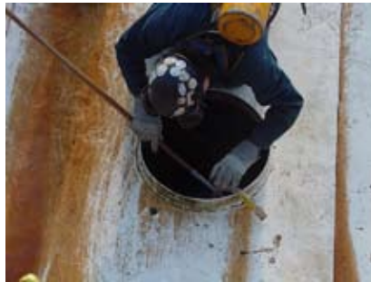
Air inlet is fished out from roof with a handle.
