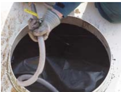
Air line is connected.
