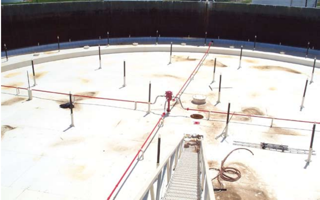
Foam Delivery System: View from floating roof showing radial piping and foam manifold
